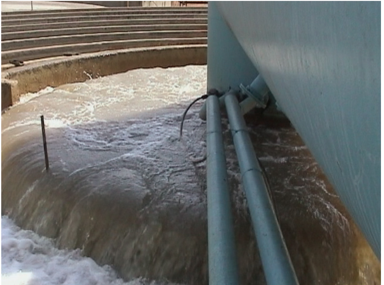
Figure B1.5: Hydraulic rapid mixing at Vereniging works of Rand Water.
